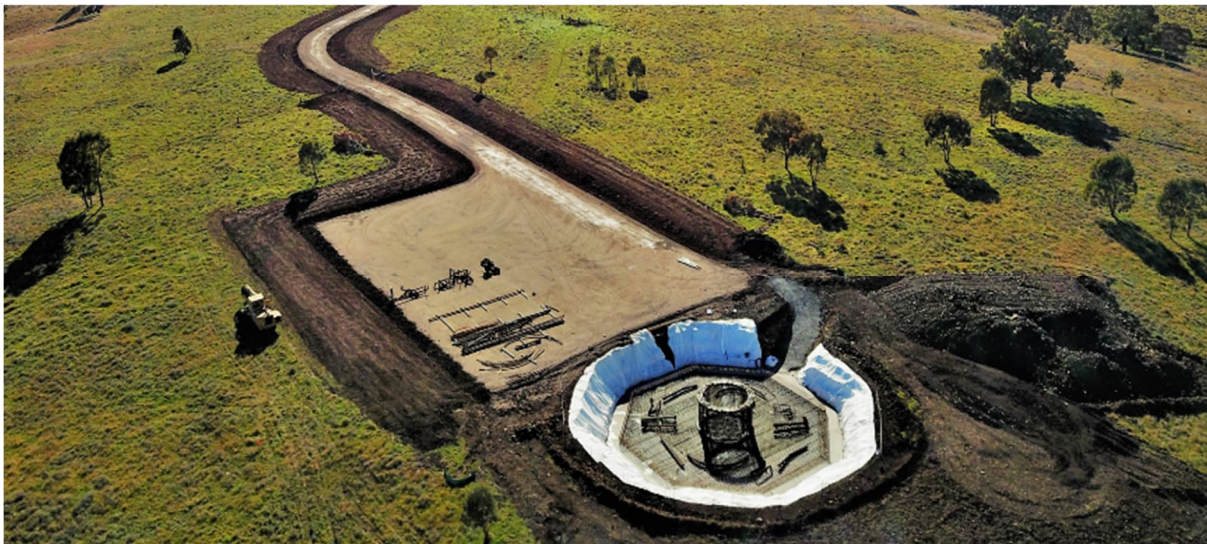
Photograph 5.6: Photo of a hardstand area, foundation and integrated crane pad and blade assembly area, with access via a spur road.
