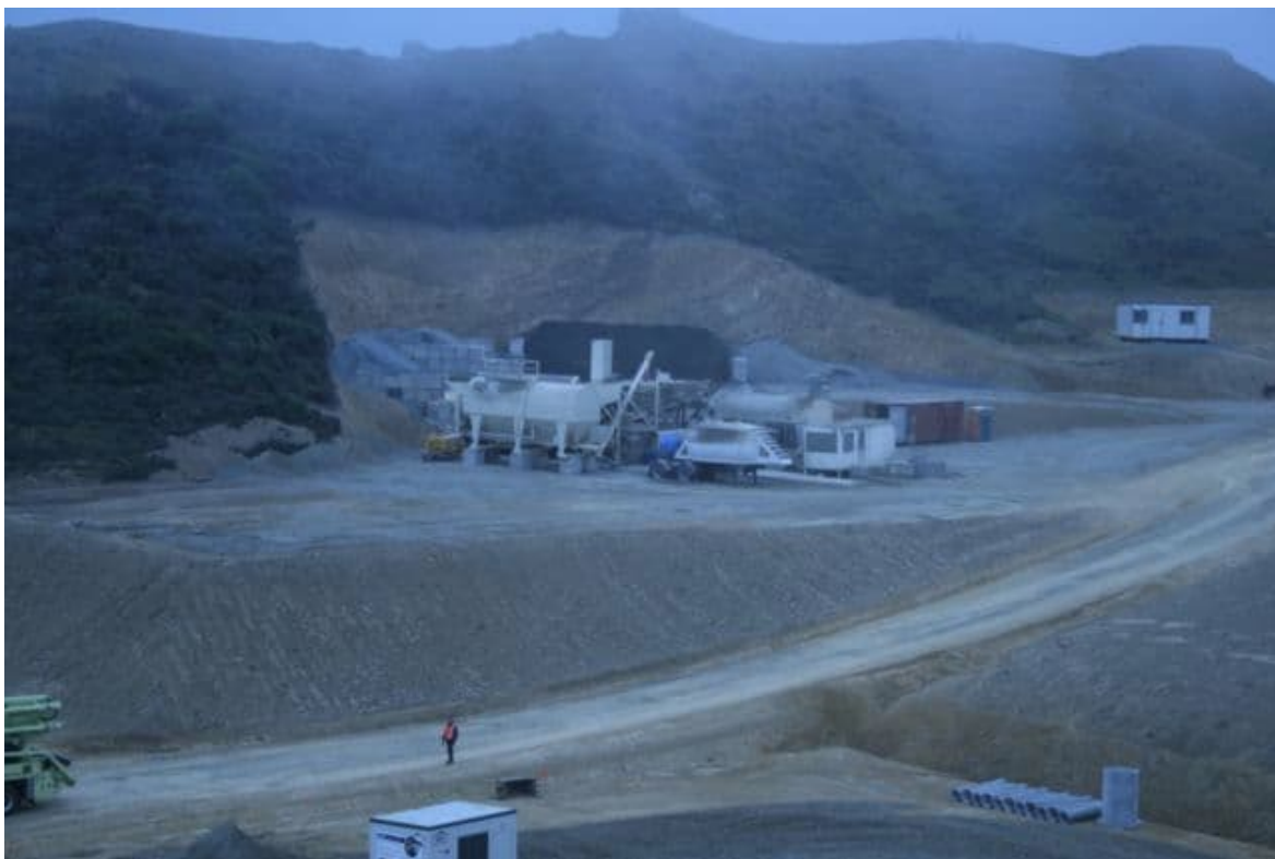
Photograph 8.1: Typical mobile concrete batching plant
